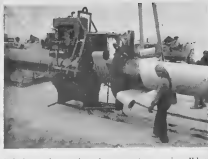
Painting and wrapping pipe prevents corrosion. When pipe was ready to be buried, machines such as this painted it with special asphalt coating, then wrapped it in heavy kraft paper and glass fiber fibers.
